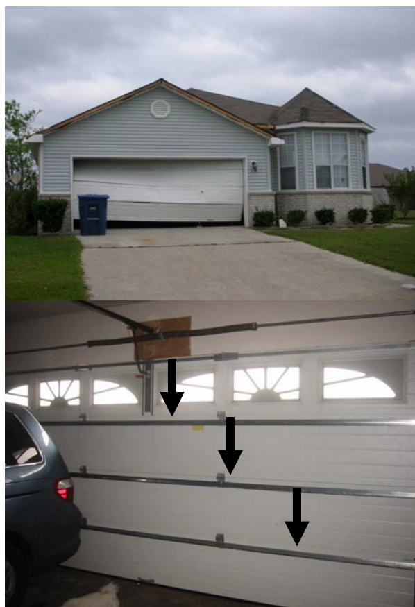
As can be illustrated from the above photo, taken near Biloxi, Mississippi after Hurricane Katrina, garage doors—especially wide garage doors—are very susceptible to wind damage, often buckling from the force. The photo was taken by an engineering professor from the University of Western Ontario while doing damage surveys for an ICLR project. Horizontal steel bars were added to the garage in Edmonton to prevent such a failure from occurring.
