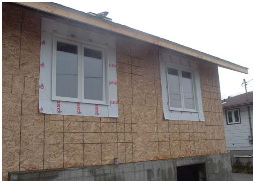
Ontario's first-ever Safer Living home was constructed in Sudbury. The house, a partnership between ICLR and The Co-operators, was built after the family's original homestead was destroyed by fire.
