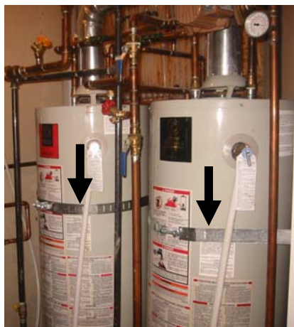
The home's hot water tanks were strapped to the walls to guard against water damage and gas leak/explosion, should they be jarred loose from their anchors.
