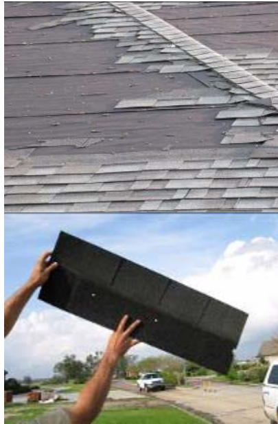
Close-up photographs showing typical shingle failures with the nails still in the roof (top) and one of the shingles that came off with two nail holes visible (bottom).
